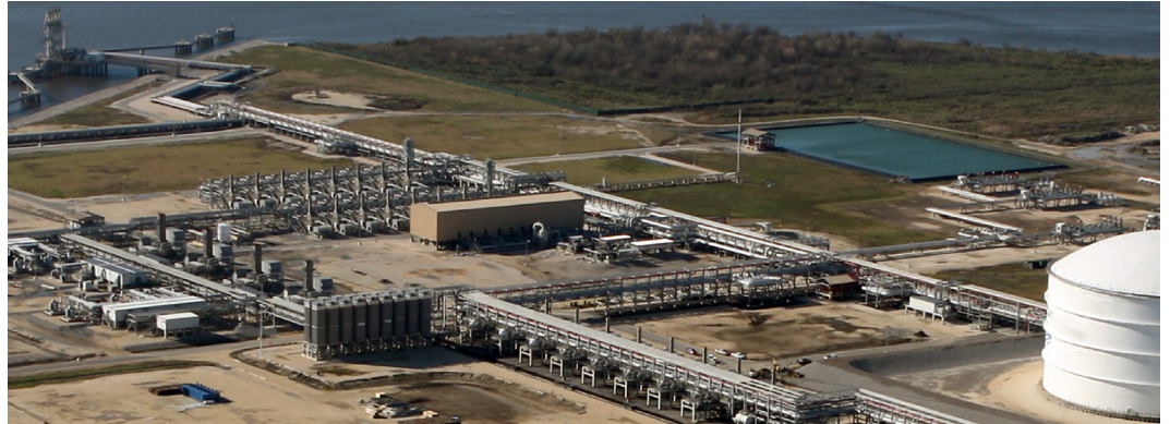
24 Sub-X ® 120-186 MM SCFD SCVs installed at a US Gulf Coast LNG import terminal
