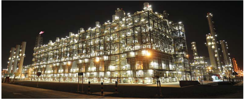
Ethylene furnaces supplied on an EPC basis by Linde Engineering North America Inc.
