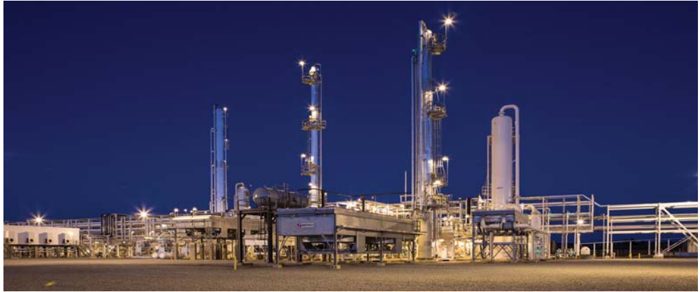
200 MM SCFD natural gas liquids (NGL) recovery plant.
