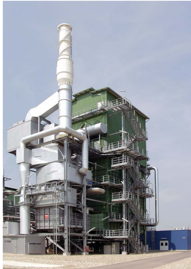
Reformer and Convection Section
