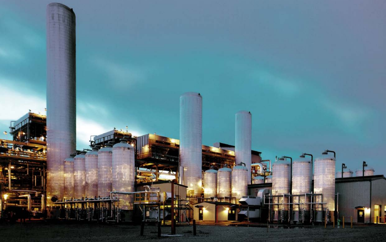
Two pressure swing adsorption units in Canada
