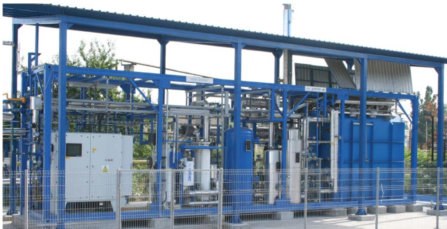
Fully modularized HYDROPRIME® hydrogen generator.
