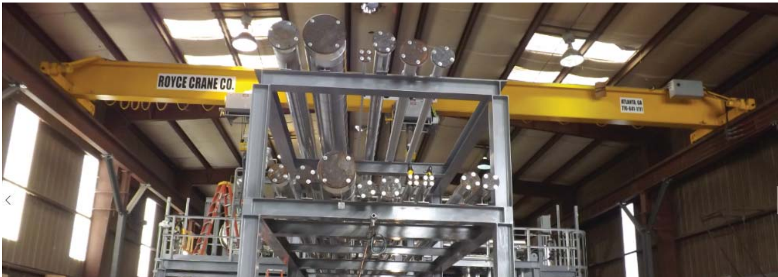
Pipe rack and 15-ton bridge crane.
