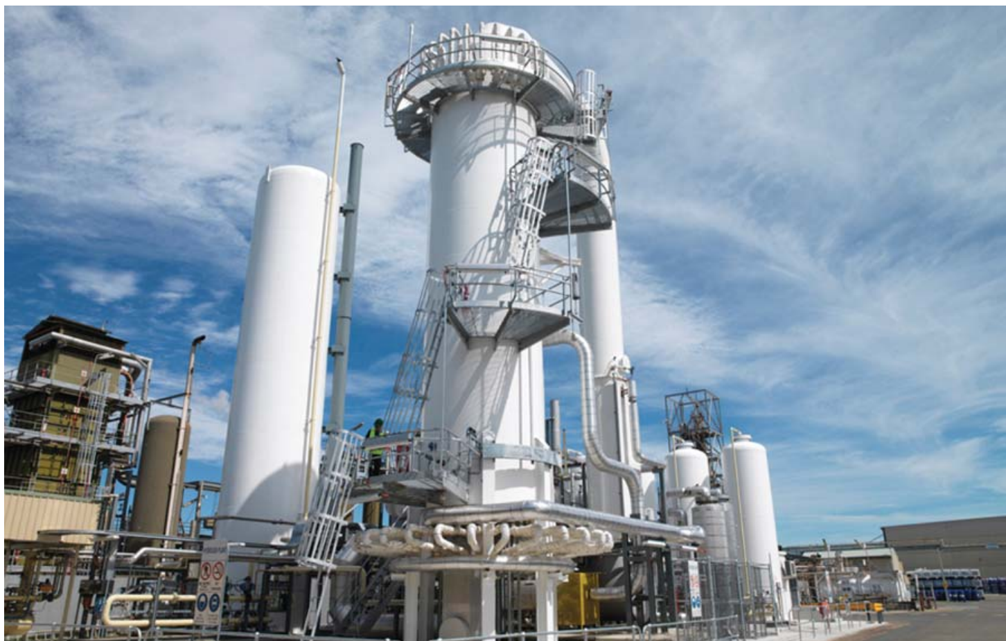
Hydro-Chem modularized hydrogen plant, fabricated and modularized in our facility.
