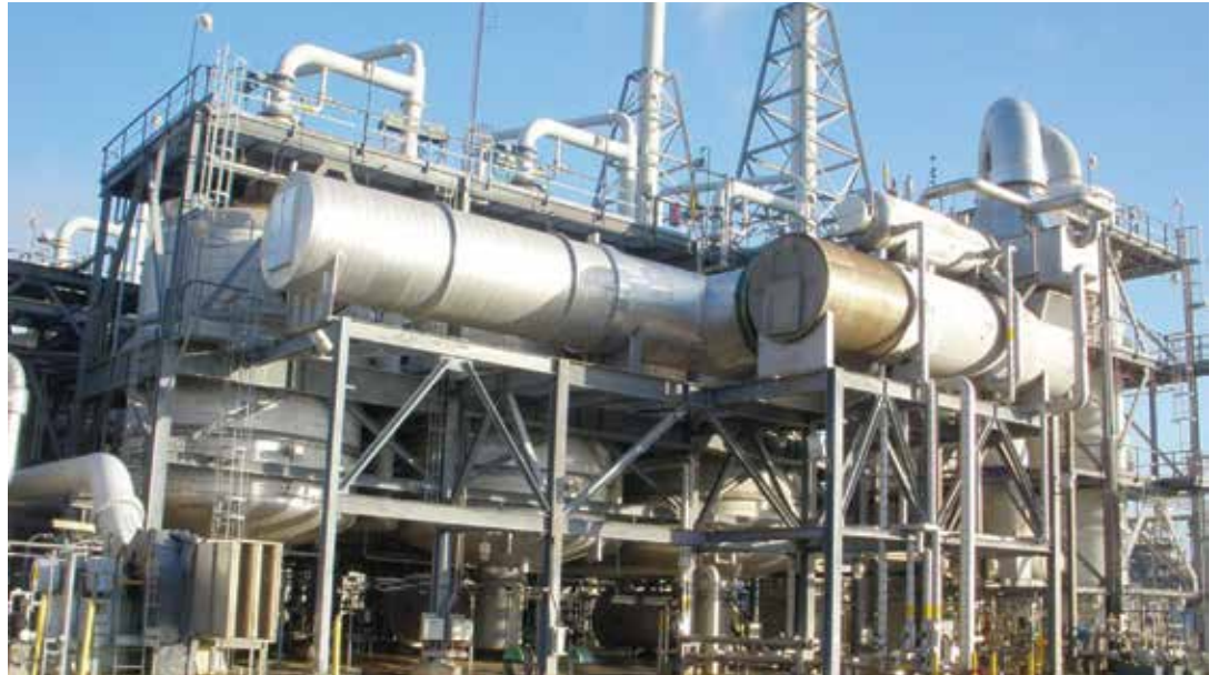
Flameless oxidizer system at a petrochemical plant.
