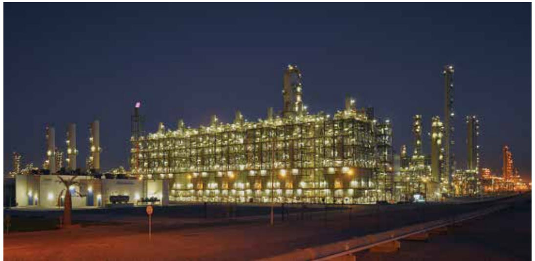
Seven ethylene furnaces supplied in United Arab Emirates
